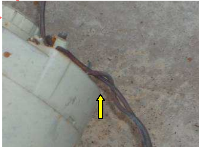
Improper ground connection
