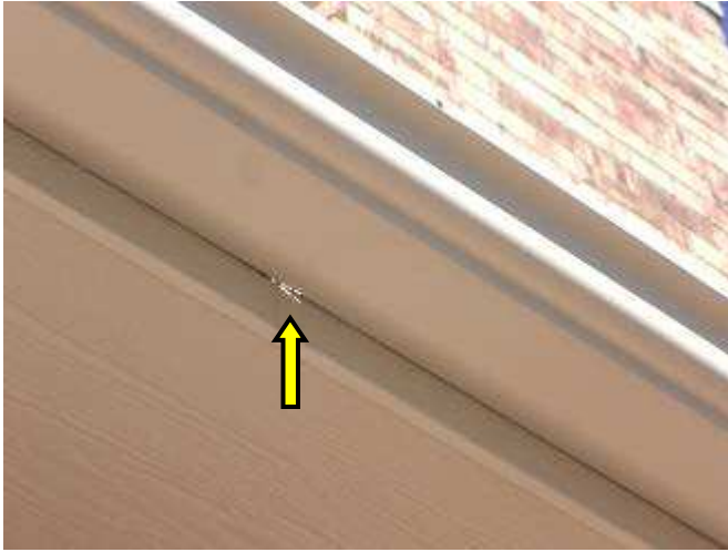
Hole in gutter
