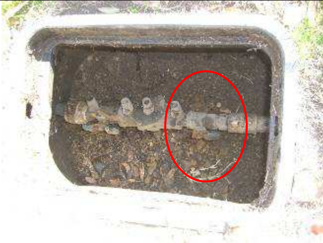
Handle rusted away
