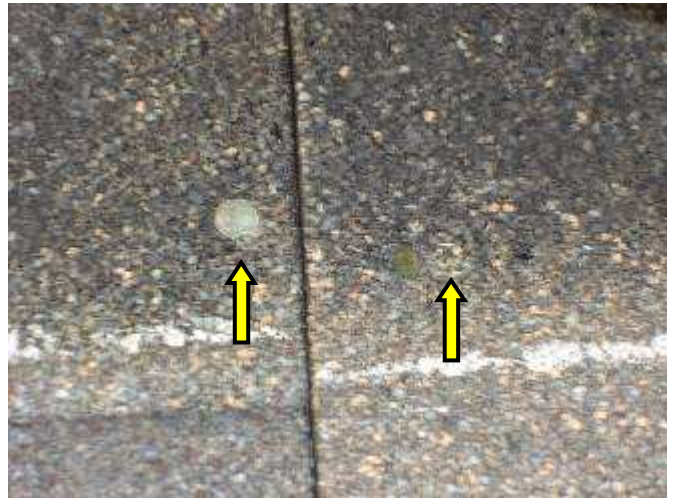
Nail over driven Nail too close to edge
