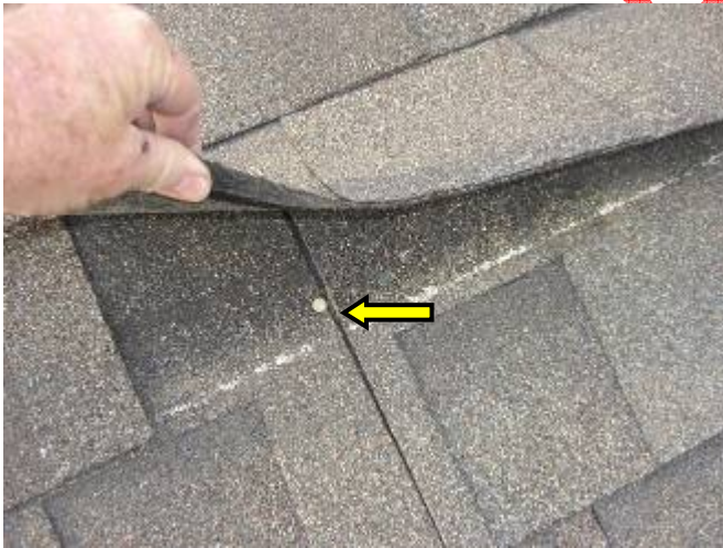
Nail too close to edge of shingle Nail above nail line
